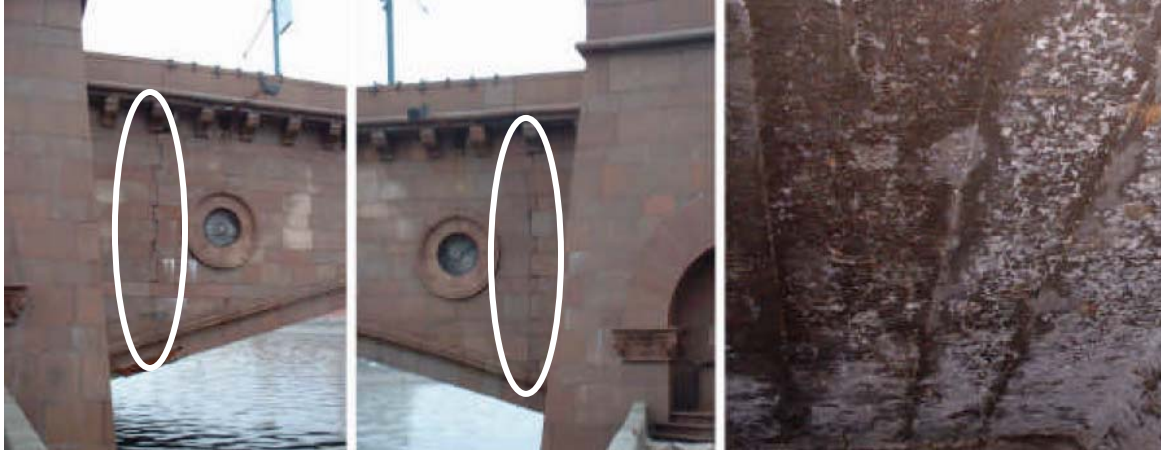
Fig. 3. Cracking of the stone walls (ellipses on left photos) confirms the settlement in the middle of the arch; penetration of chlorides is visible in the interior of the arch boxes (right photo).
